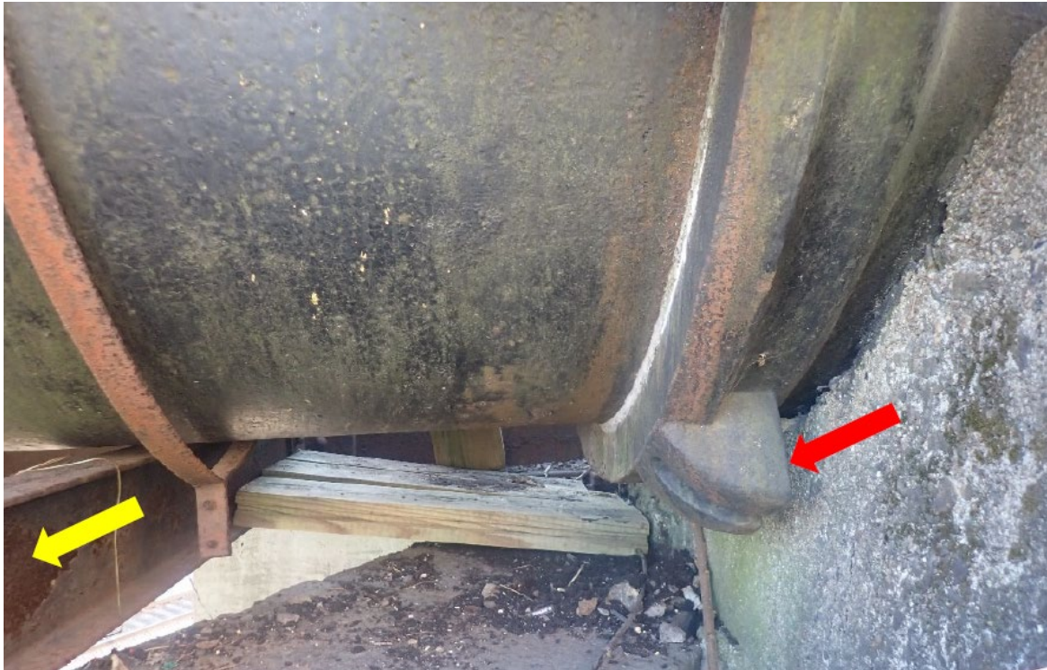
Attachment point for missing rod highlighted with red arrow. Obstructing structural member highlighted with yellow arrow.
